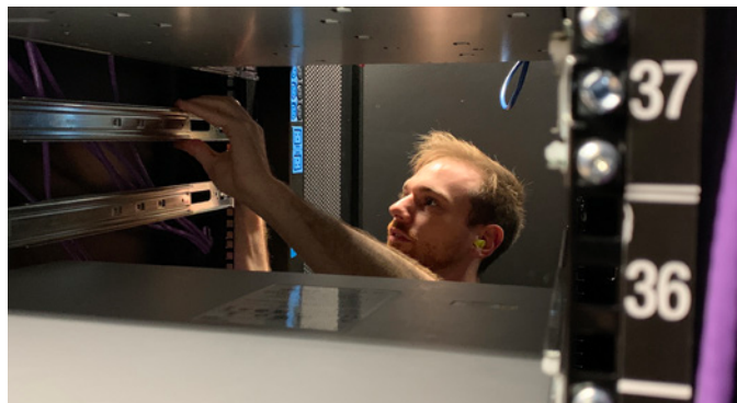
Shockbyte deployed AMD CPUs to bring its bare metal deployment in house.
